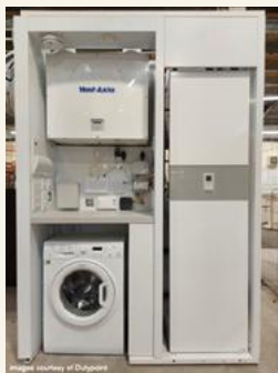
Example utility cupboard connected to the energy sharing network.
